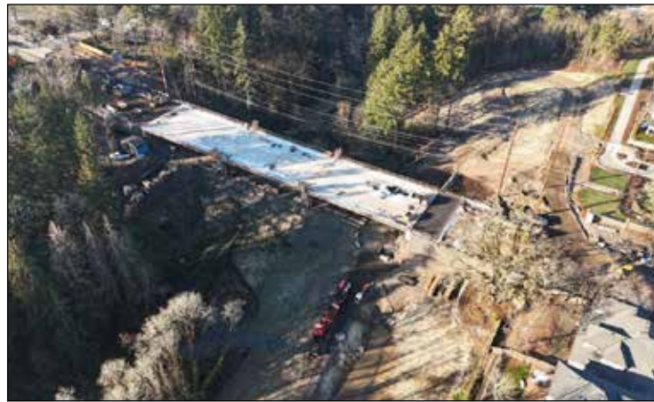
This birds-eye view looks north at Boeckman Road, where the Boeckman Bridge foundation, girders, diaphragms, abutments, and deck are now complete.
